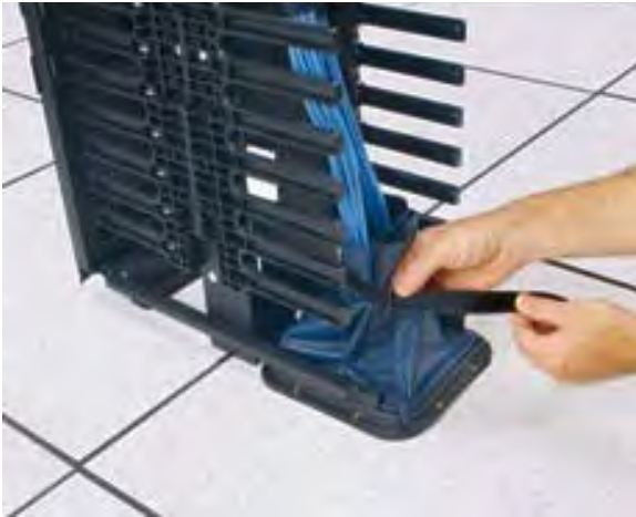
Figure 14-18 Gasket Seals Off Access Floor Tile Cutout In Vertical Cable Manager
