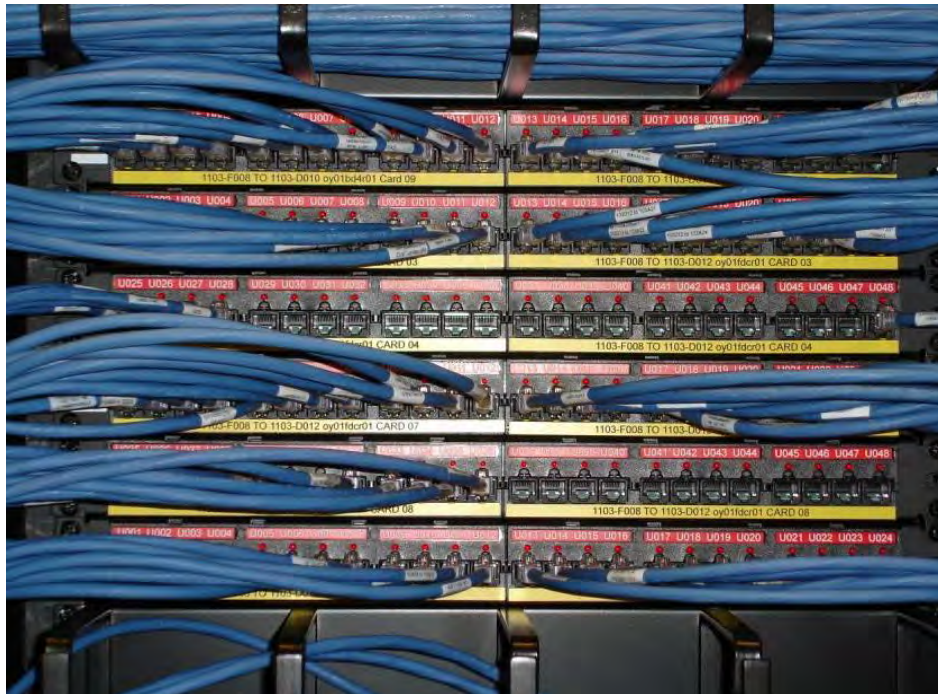
Figure 14-15 Example of Labeled Termination Ports and Equipment Cords
