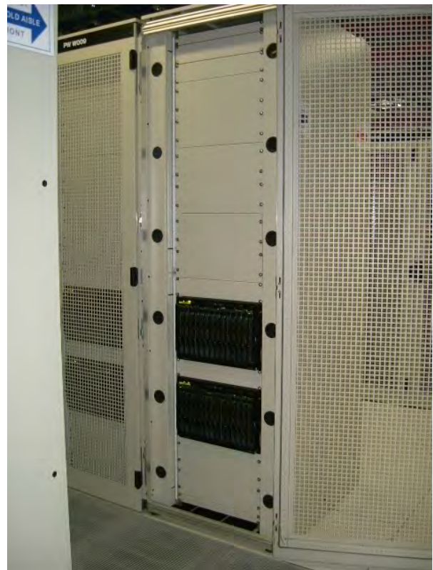
Figure 14-11 Blank Panels Installed in Empty RUs
