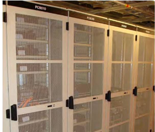
Figure 14-14 Cabinets Are Identified and Labeled
